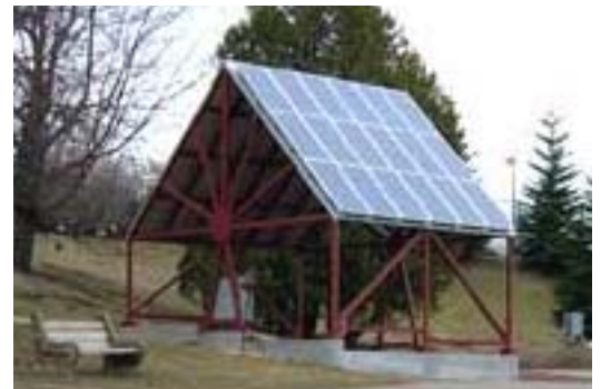
Solar panels at the Duluth Zoo.
