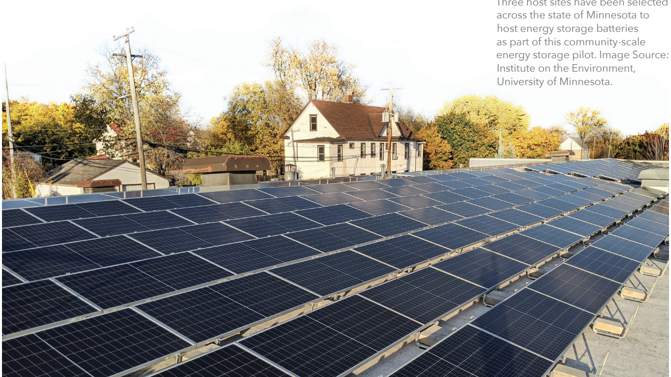
North Minneapolis, Minnesota. Renewable Energy Partners solar installation site.
